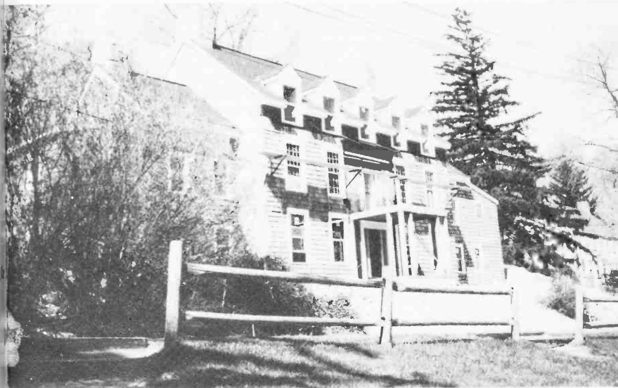
The new Williams House, built with LIBA contributions, nears completion in spring 1977.
